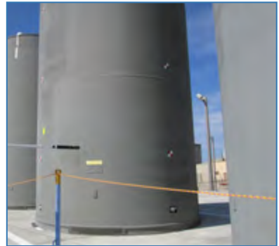
Dry canister storage
